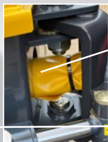
Protected hose lines
